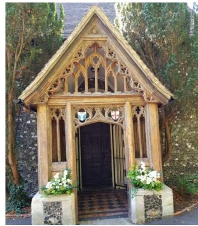
Ledges on North porch
